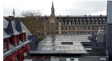
40kW scalable xStorage Buildings system at the Catholic university of Lille, France
